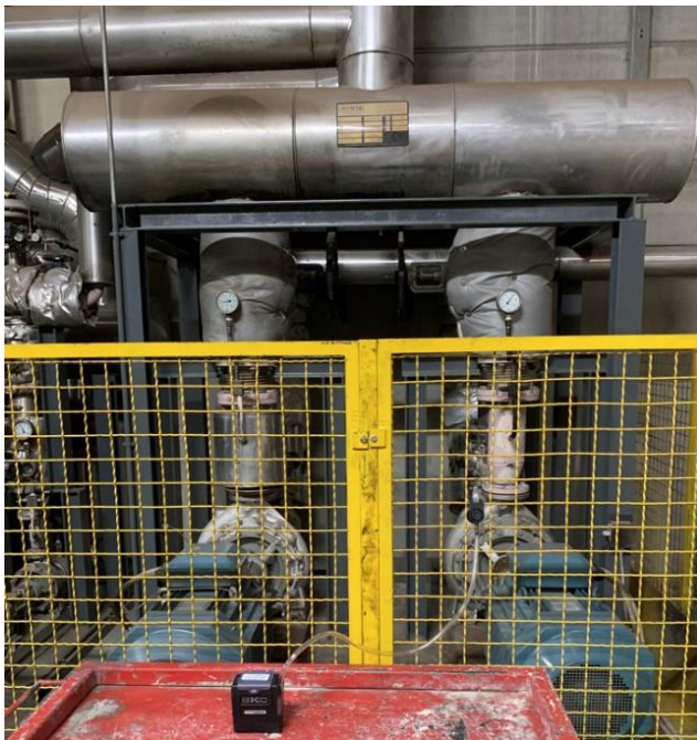
Figure 11. Air sample point in Site S-08
