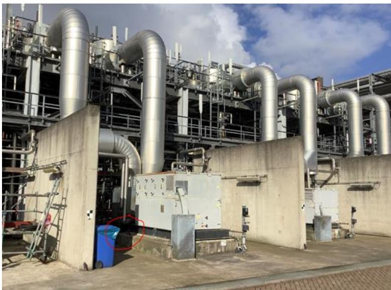
Figure 5. Air sample point in Site S-02
