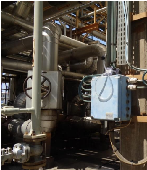
Figure 10. Air sample point in Site S-07
