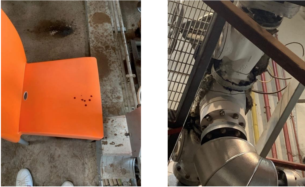
Figure 9. Terphenyl, hydrogenated leakage and leakage point at Site S-06
