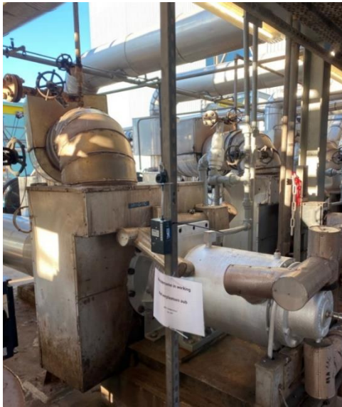
Figure 12. Air sample point in Site S-10
