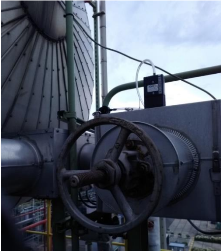
Figure 7. Air sample point in Site S-05
