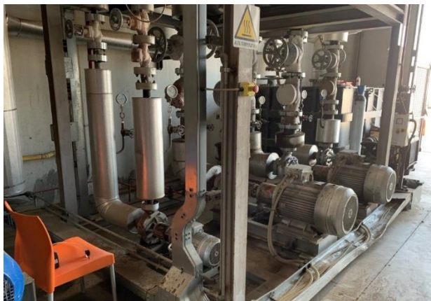
Figure 8. Air sample point in Site S-06
