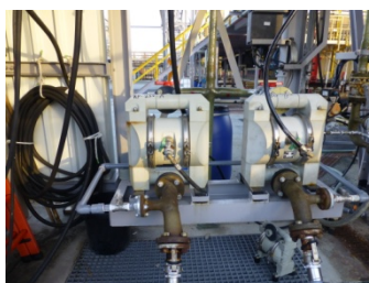
Pumps with flush lines
