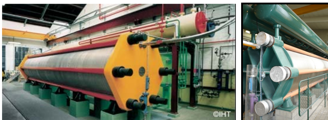
Four cellblocks mounted together, IHT construction on the left and AAK on the right
