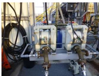
Pumps with flush lines
